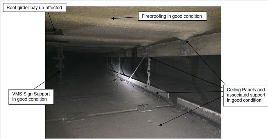
Photo 3. General View of Exhaust Plenum – no signs of fire related dis-stress
