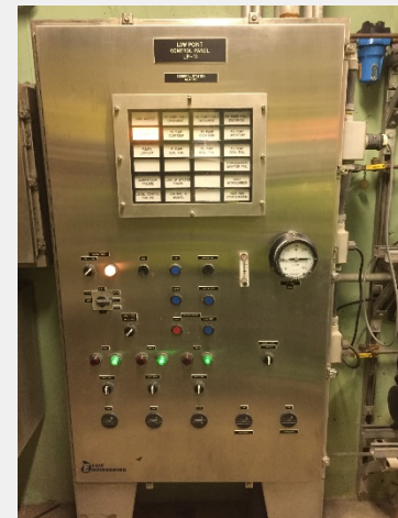
In-field pump controller alarm
