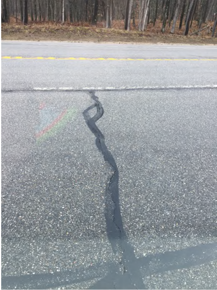
Should have been routed
