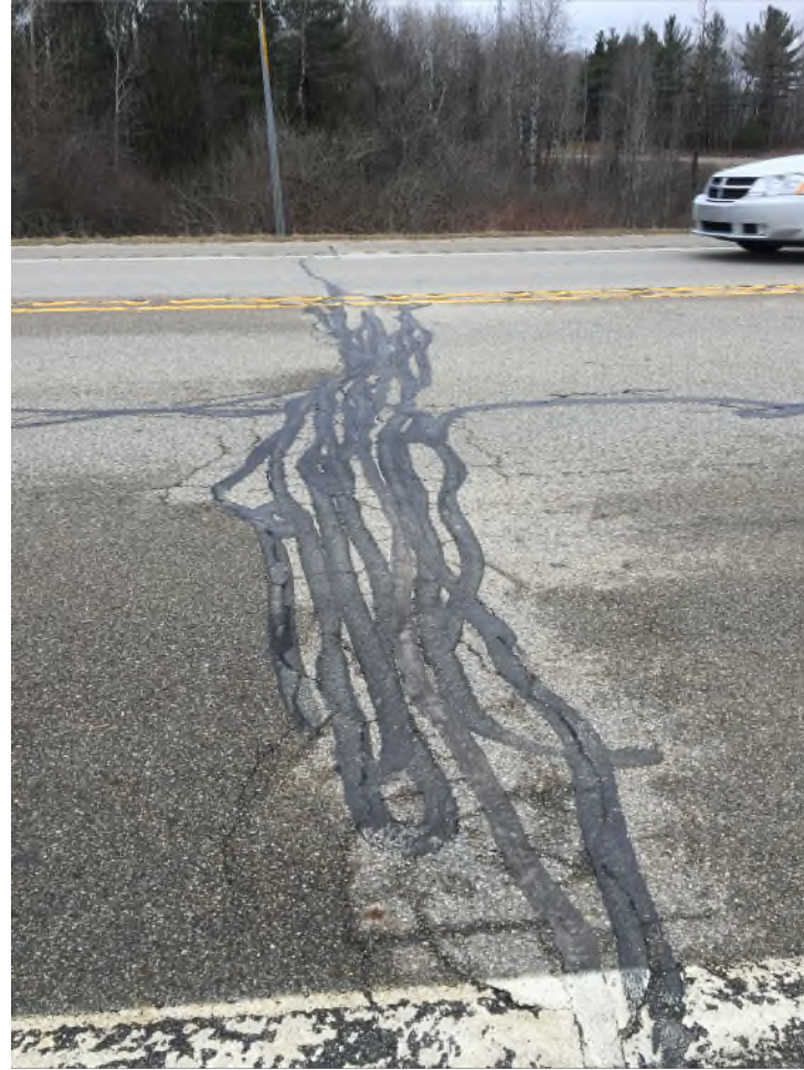
Multiple cracks in composite
