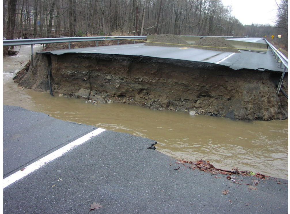
April 2005 Flood SR 209 Ulster Cty, NY
