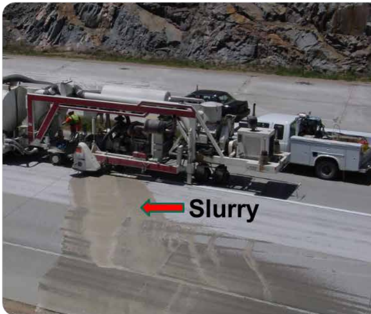
Slurry Recovery Failure
