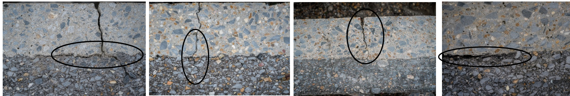
(a) Crack initiating debonding (b) Crack propagating to AC (c) Saw cut joint cracked through (d) Debonding at interface
