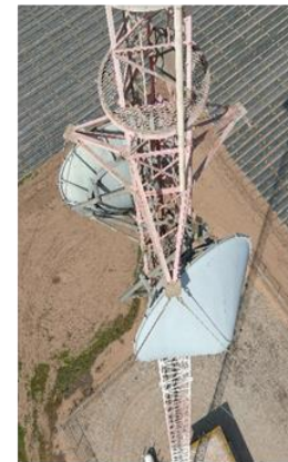
SNS RCLR Comms Tower
