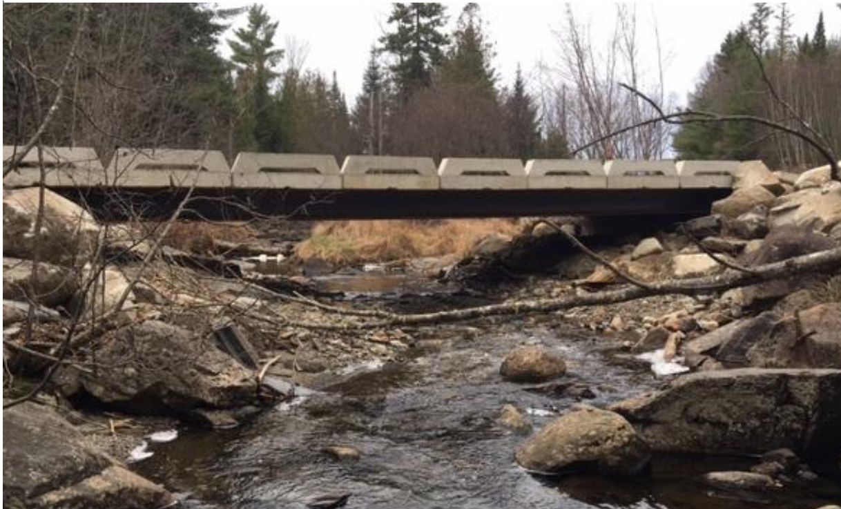
Fish- and wildlife -friendly resilient bridge, Abbot Village, Piscataquis County, Maine. Source: USDA - Natural Resources Conservation Service, photo Ben Naumann
