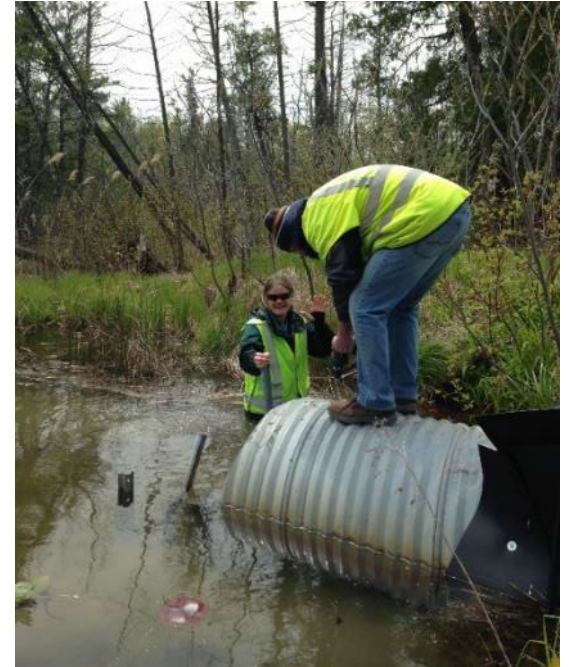
Existing drainage culvert used by freshwater turtles Photo Credit: Ausable Bayfield Conservation Authority
