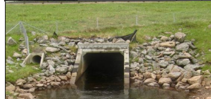
Round pipe culvert top left with drainage culvert (Jochen Jaeger)
