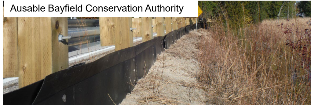
Plastic attached to guard-rail
