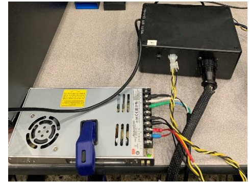
Power supply and control box
