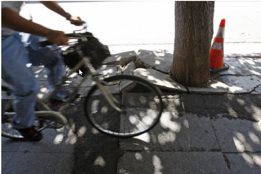
A buckled sidewalk at 4th and Main streets in downtown L.A. (Gary Friedman / Los Angeles Times)
