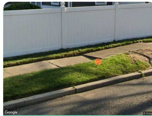
Surface Problem Severity ●●●●● Tags uneven/slanted
