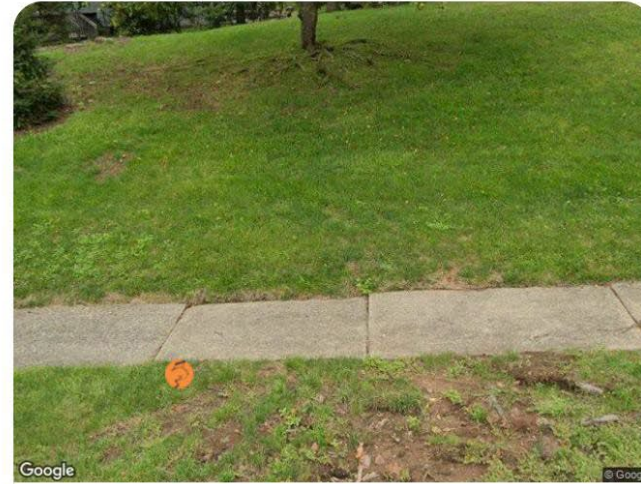
Surface Problem Severity ● ○ ○ ○ ○ ○ Tags uneven/slanted height differ..
