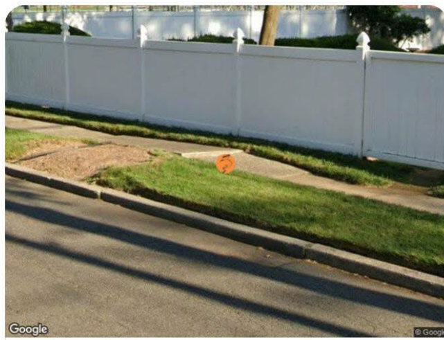
Surface Problem Severity ●●●●● Tags uneven/slanted
