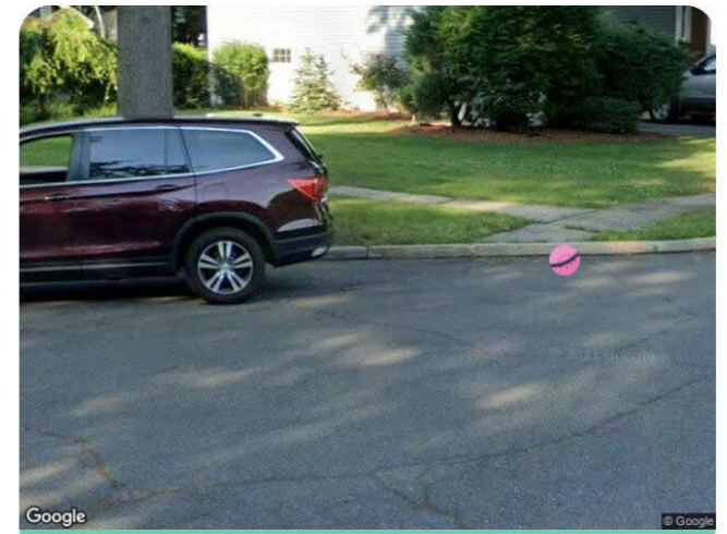
Missing Curb Ramp Severity ●●●●●○
