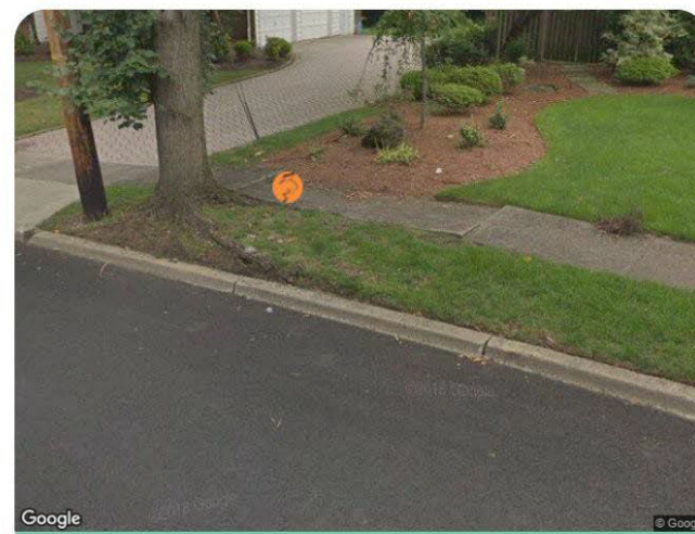
Surface Problem Severity ●●●●● Tags uneven/slanted height differ... +1
