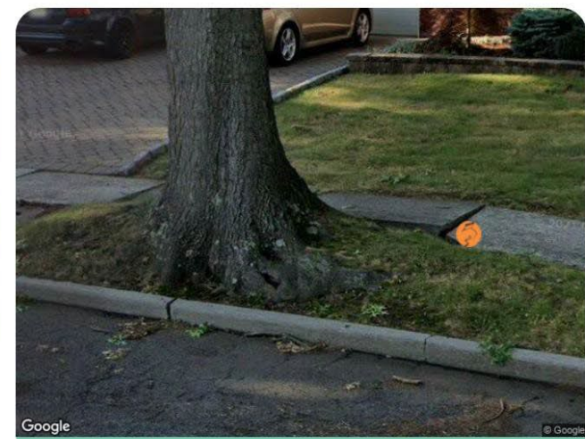
Surface Problem Severity ●●●●● Tags uneven/slanted
