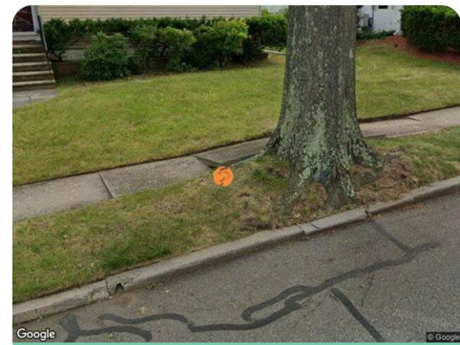
Surface Problem Severity ●●●●● Tags uneven/slanted
