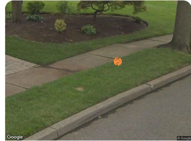
Surface Problem Severity ● ● ○ ○ ○ ○ Tags uneven/slanted height differ..
