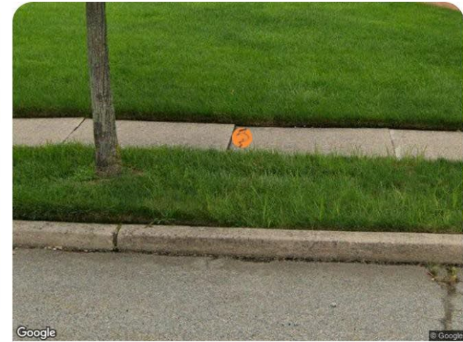
Surface Problem Severity ● ○ ○ ○ ○ ○ Tags height difference
