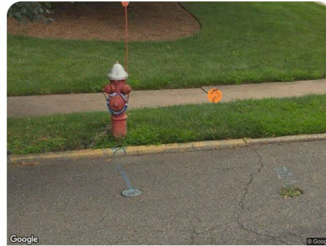
Surface Problem Severity ● ○ ○ ○ ○ ○ Tags cracks height difference
