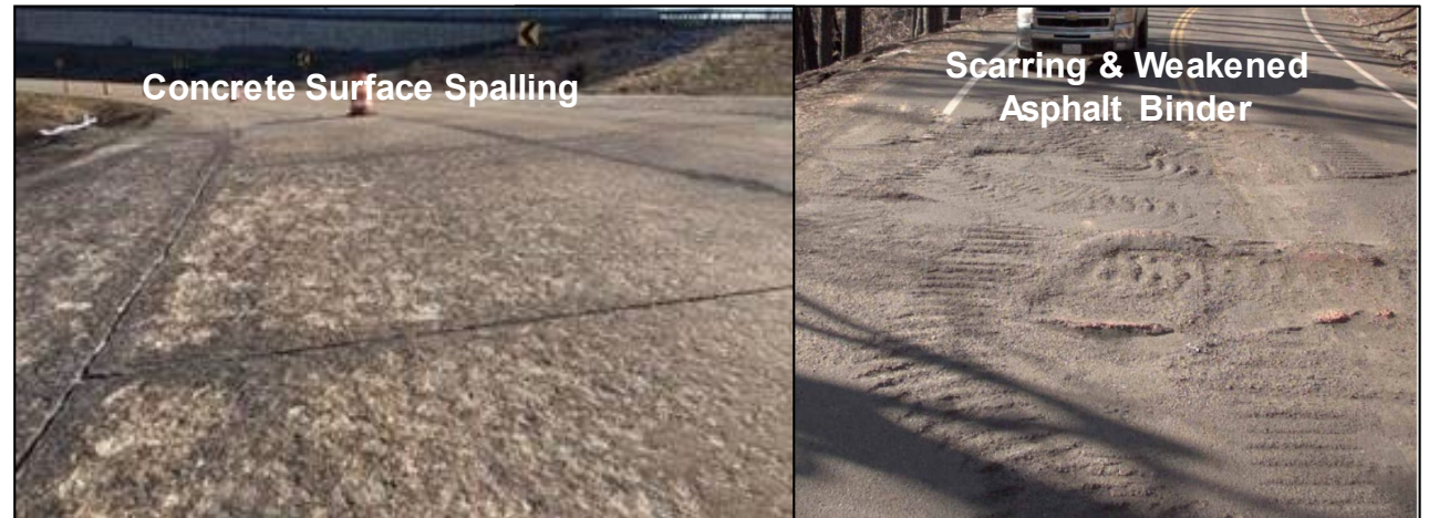
Pavement Damage due to Car Fires
