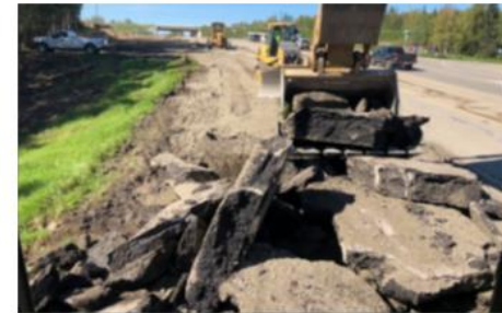
In some places, up to 12 feet of old patched asphalt had to be removed.
