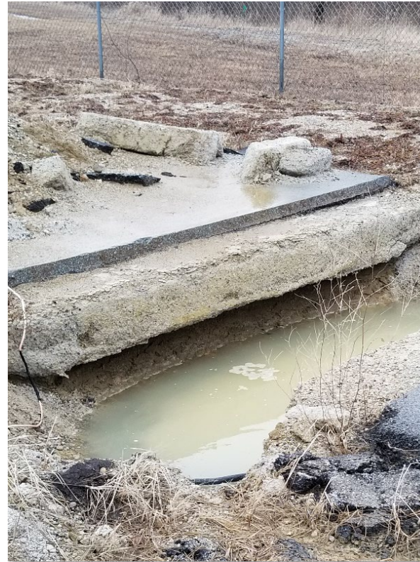
C2S1 Eroded Subgrade, intact base
