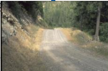
a. Overflow dip protection at a fill stream crossing. (Adapted from Weaver and
