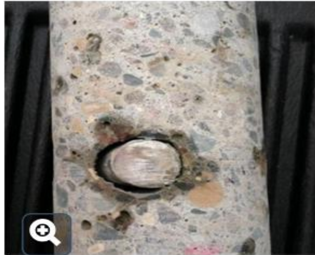
Unacceptable Grout Adhesive Coverage
