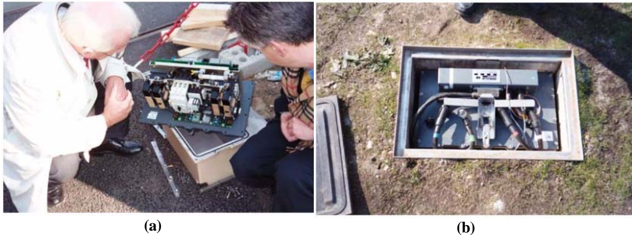
FIGURE 13 (a) Interior of power rail control unit; and (b) Installed power rail control unit.
