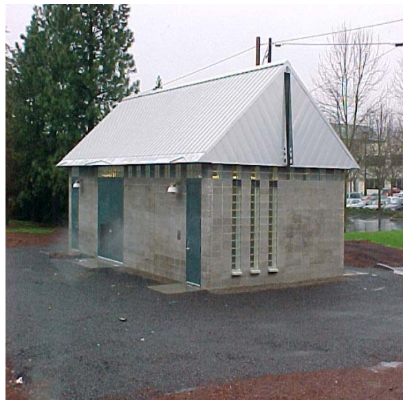
FIGURE 8 TriMet Interstate MAX LRT Failing Street Substation, 2003.
