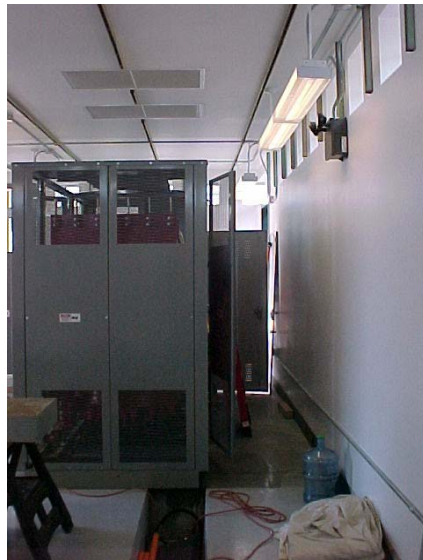
FIGURE 10 TriMet Interstate MAX LRT Expo Substation, 2003.
