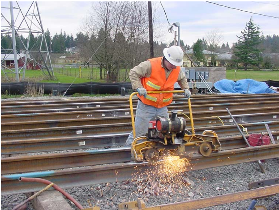
FIGURE 6 Interstate MAX light rail construction worker grinding string with profile grinder at Ruby Junction Maintenance Facility Expansion Project.
