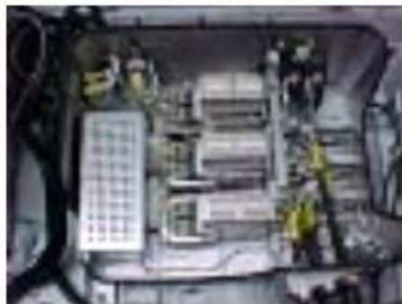
FIGURE 18 Power control box.
