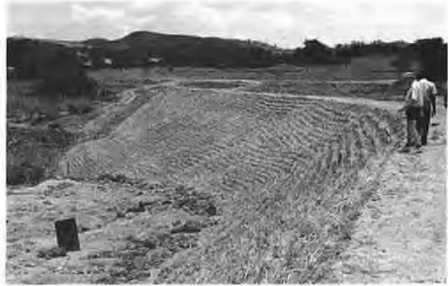
FIGURE 11 Newly planted vetiver on downstream slope of earth dam in Zimbabwe. Vetiver rows have actually been planted too close together and are therefore more costly than necessary. Lines should have been planted about 1 m apart (photograph courtesy J. C. Greenfield).
