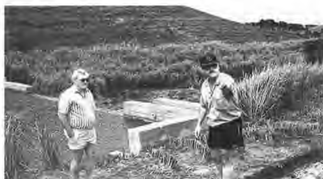
FIGURE 13 Vetiver stabilizing concrete-earth interface and protecting sides of downstream drainage way, Natal, South Africa (photograph courtesy J. C. Greenfield).
