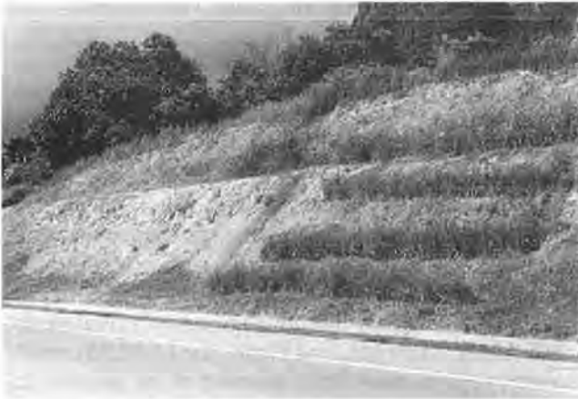
FIGURE 5 Malaysia test planting using containerized raised plants on highway cut 8 months after planting vetiver hedges. Note unprotected area continues to erode; where protected, other grass species are now able to become established. Alternative to vetiver is to continue applying costly and often ineffective hydroseeding techniques (photograph courtesy P. K. Yoon).
