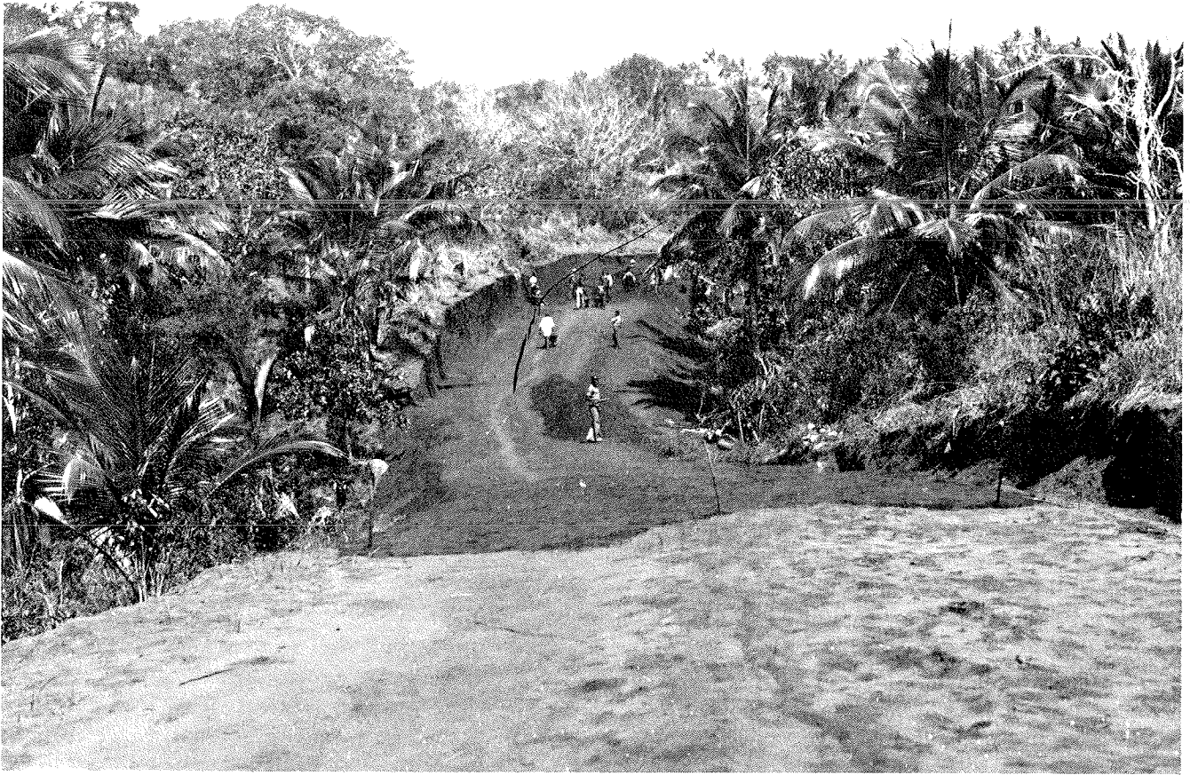
xxviii Labor-Intensive Rural Access Roads Programme in Kenya uses long-term environmental compaction before reshaping and applying surfacing material (photo courtesy of TRRL, United Kingdom).
