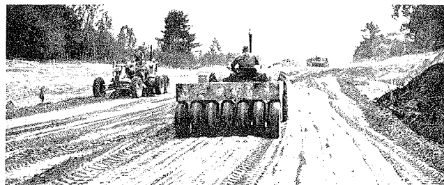
STAGE COMPACTION —An unballasted machine often makes the first pass on loose, high lifts to form crust for heavier rigs that will bring soil to specifications.
