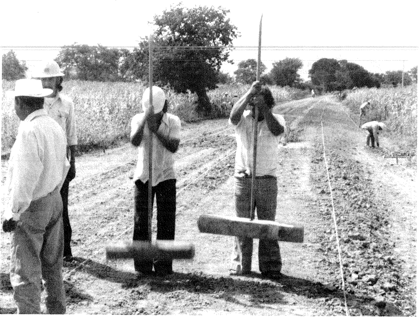
String lines define proper crown and grade of single-lane, labor-intensive embankment construction; final compaction occurs under traffic load (Mexico).
