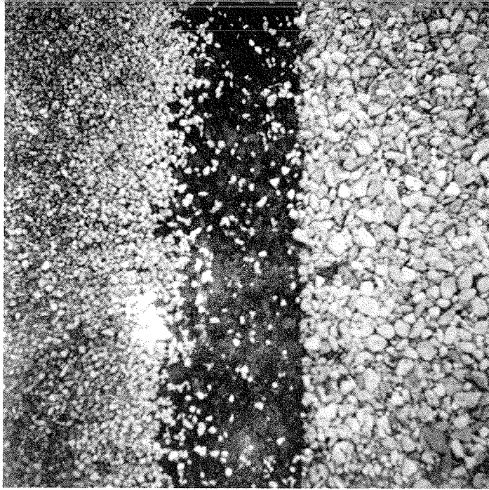
Fig. 30. Illustrating Coarse Aggregate Used for the Bottom Layer on the Right and Finer Aggregate on the Left for the Top Layer of a Double Surface Treatment, Together with a Portion of the Second Application of Asphalt Binder.
