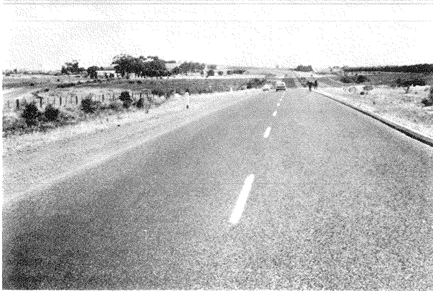
Fig. 6. Victoria, Australia. Single Surface Treatment on Consolidated Granular Base on 4-Lane Divided Highway between Melbourne and Sydney--the Hume Highway Near Melbourne, 6 Years Old, Carrying 4000 Vehicles per Day.
