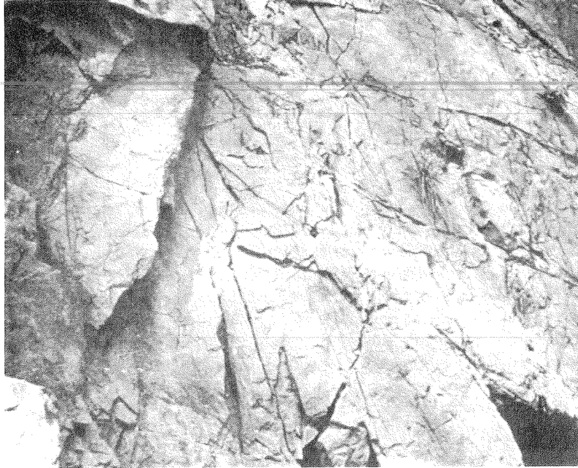
Fig. 22 Cracks in stiff fissured clay
