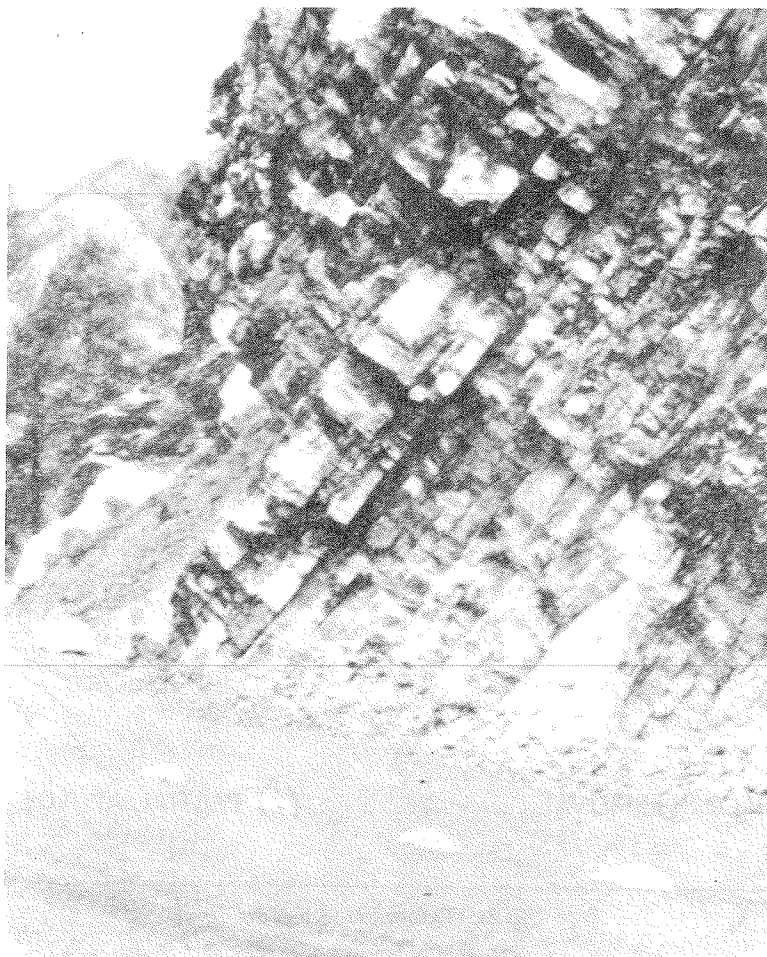
Fig. 33 Dip favourable for the road and unfavourable for the same road beyond the turning
