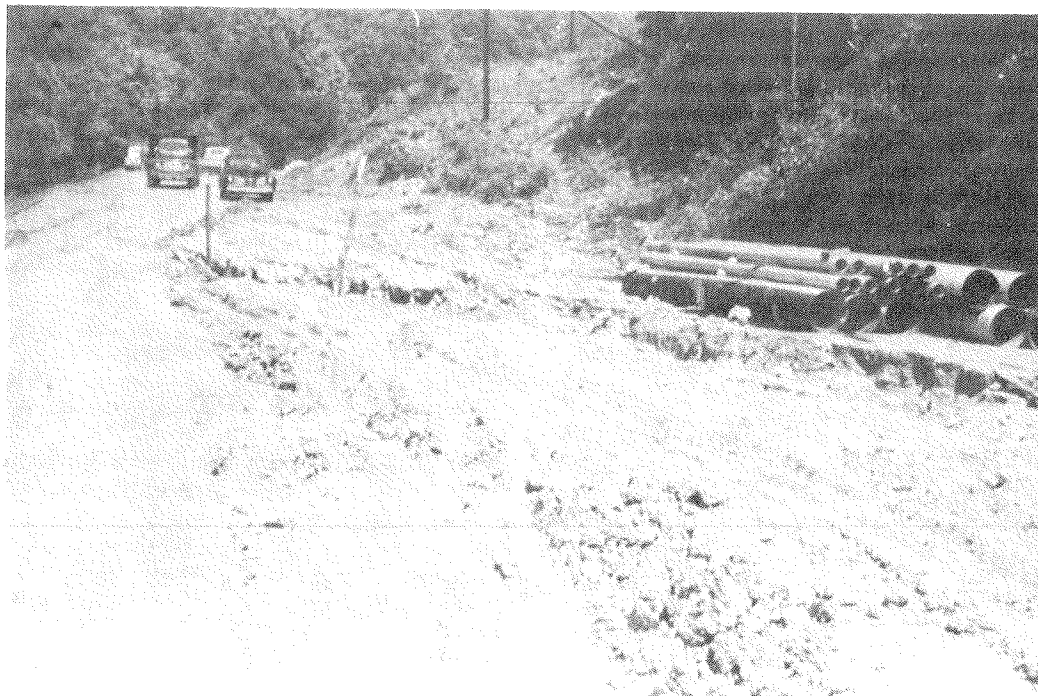
Figure 11. Photograph of roadway in Kanawha County near Charleston, West Virginia. Note break at right edge of picture.
