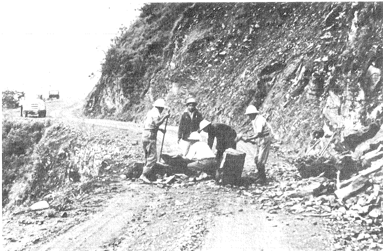
Cover photo: Slide-prone areas cause maintenance problems in Bolivia.
