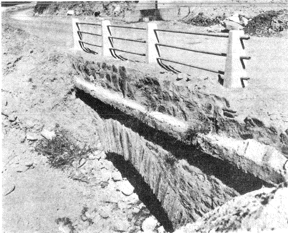
Fig. 36 Culverts clogged up due to poor maintenance practice
