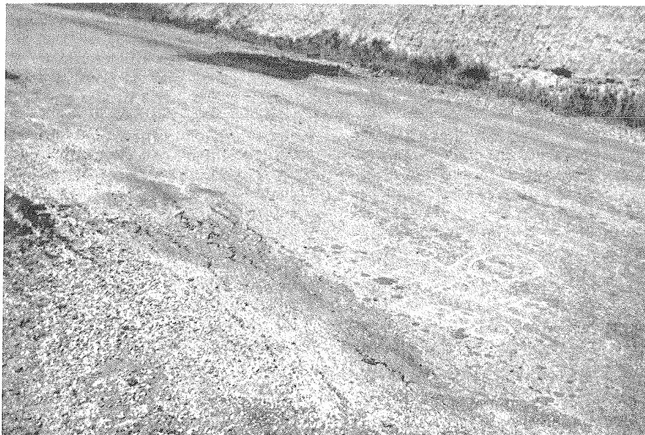
Figure 15. Poor Performance of Flexible Pavement Constructed on Clay Shales of the Northern Great Plains, Near Glendive, Montana - Lebo shales are similar to those illustrated in Figure 14.
