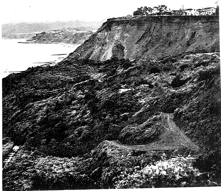
Figure 1.—Stump-type landslide which covered U.S. Highway 101 at Pacific Palisades, Los Angeles County, Calif. (Courtesy California Division of Highways.)
