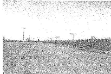
Figure 23. Flexible Pavement Constructed on an Ohio River Granular Terrace, Switzerland County, Indiana (20) - Only very shallow side ditches are required because of good internal drainage of the terrace materials. Highways on granular terraces usually give excellent performance.
