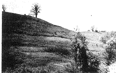
Figure 8. Sloughing of Colluvial Hillside - Eastern Ohio County, Indiana (10) - Rock and soil break away from the hill to produce landslides.
