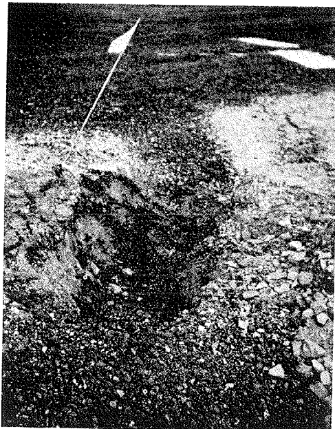
Figure 20. Progressive Failure Results in Deep Caving
