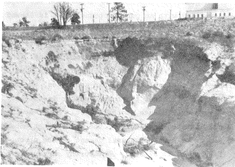
Figure A2. Failure of outlet structure due to gully scour
