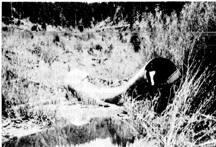
Fig. 20—Culvert and roadway fill failure from buoyant forces. Culvert carried downstream.
