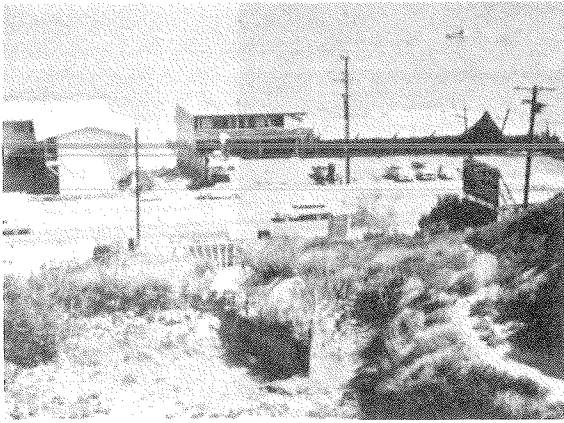
Figure 48. Debris dam and basin in foreground and steel grill debris rack at culvert entrance in background. (See Fig. 49).
