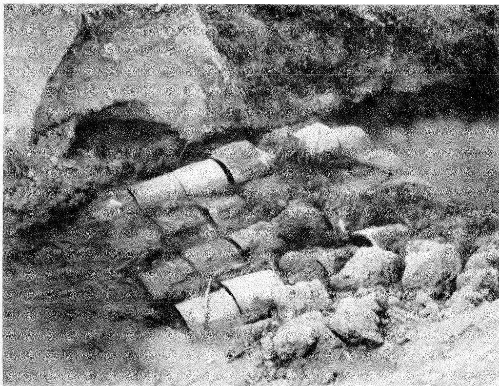
Multiple 1-m diameter concrete pipe culvert shows damage from washout—Brazil.
