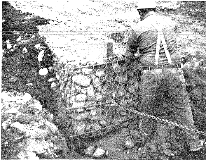
Figure 2.—Gabions Filled Under Tension. Tension (supplied by come-along) lifts baskets off ground. As they are filled, they settle back straight and true.
