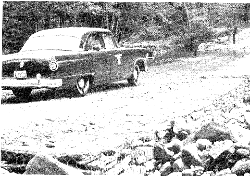
Fig. 47A — Low water bridge installed in federal forest land was built with gabions and gravel. Post marks roadway at time of high water.
