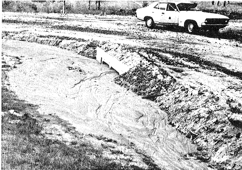
Culvert Blocked with Silt
