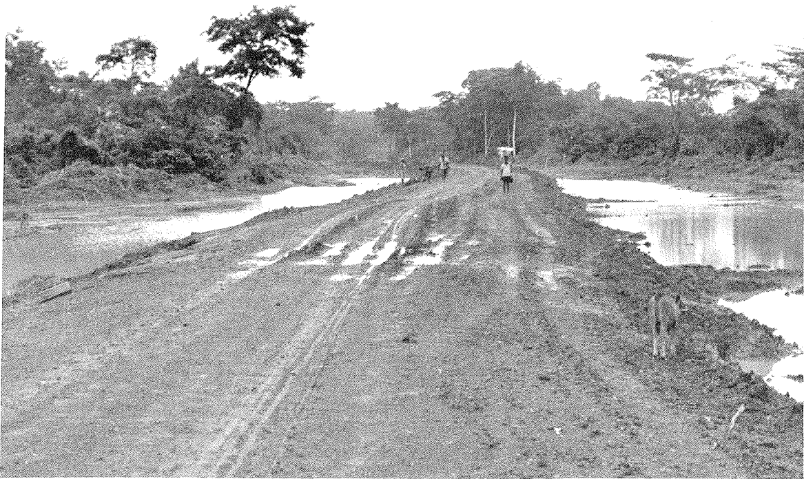
Sideborrow construction often creates standing water, a situation that requires proper ditching before road is completed (Liberia). (Photo courtesy of USAID/Liberia.)
