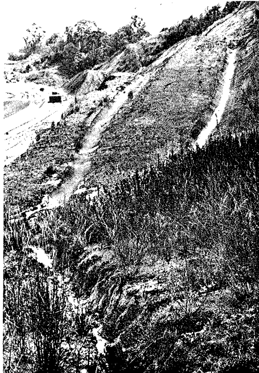
Paved and Unpaved Catch Drains
