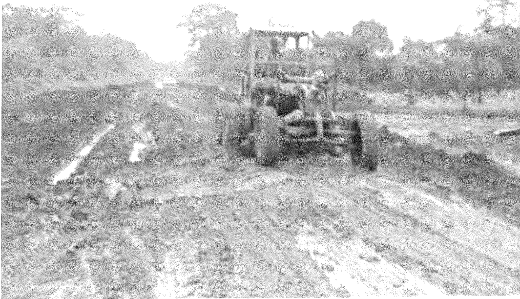
Lack of grading material for proper cross-slope during construction creates windrows at roadway's edge, causing rainfall to seep into roadbed and saturate material (Liberia).
