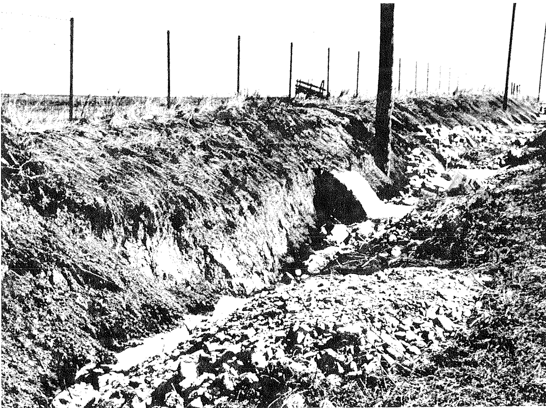
Figure 4.—Poorly designed ditch checks.
