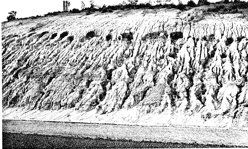
Scouring of Batter due to Lack of Suitable Drainage
