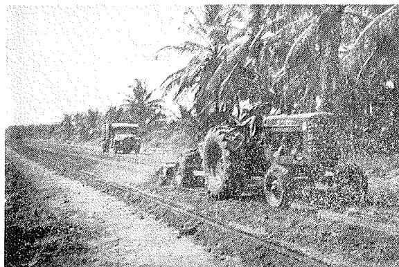
Plate 3—Final Mixing of Soil Cement and water with a Rotavator, toed to a tractor
