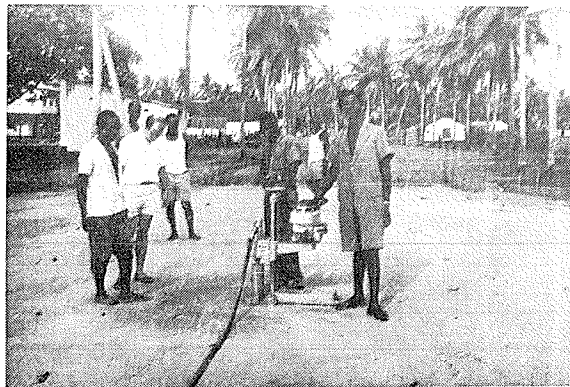
Plate 7—Cutting Cores from a finished Soil Cement road, to study the effect of age on its strength, under field Conditions.
