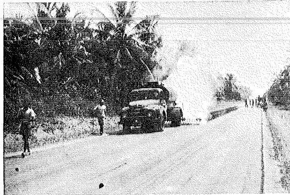
Plate 6—M. C. 2 being sprayed on a Soil Cement road soon after Compaction to act as a membrane for Curing, and a primer Coat
