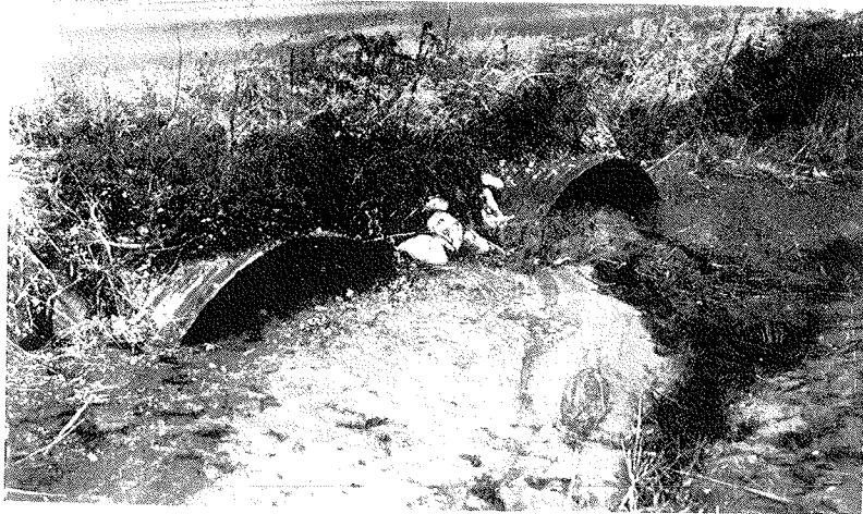
Fig. 25. This culvert is almost completely useless until it is cleaned out and the erosion which produced the silt is stopped.
