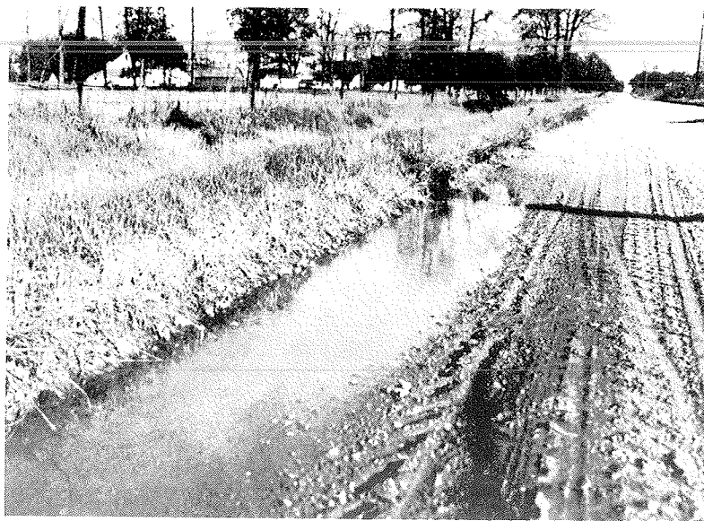
Fig. 9. This berm has no outlet. The water collected saturates and softens the roadway so that traffic creates ruts.
