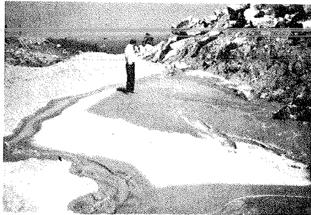
Small basins or holes on project can retain storm water and catch considerable amount of sediment. Frequent cleaning and judicious disposal of deposited materials are required.
