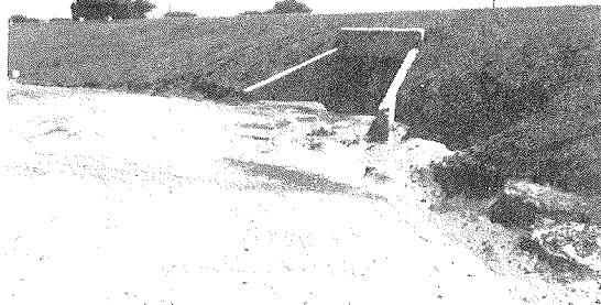
Erosion in granular fill behind unprotected culvert headwall due to streamflood conditions. Zone III Trucial Coast
