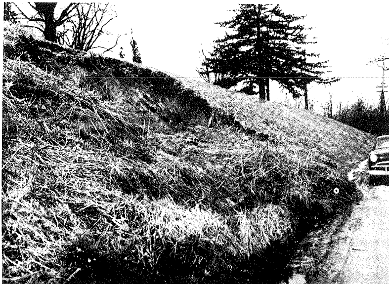
Fig. 11. No amount of grass will hold this slope which is softened by subsurface water. Subdrains must intercept the water in back of the slope to keep the soil dry.
