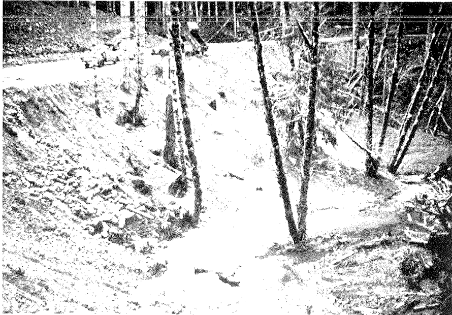
Waste material dumped over an embankment can cause serious stream pollution and kill vegetation and trees. Spoil areas should be selected with care.
