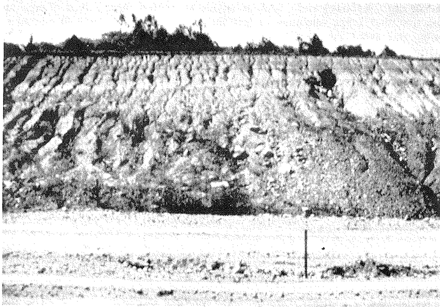
Accelerated erosion in a new cut section can cause serious downstream sediment deposits and extra costs to contractors.
