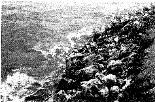
Leaching of fines from desert fill by wave action on a recently placed causeway. Arabian Gulf
