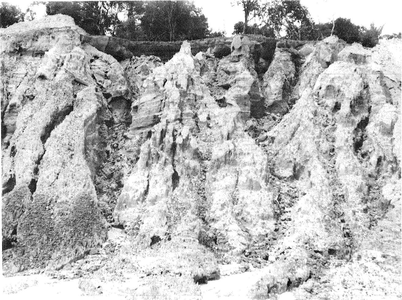
Cover photo: Eroded 8.5-m embankment (Brazil).
