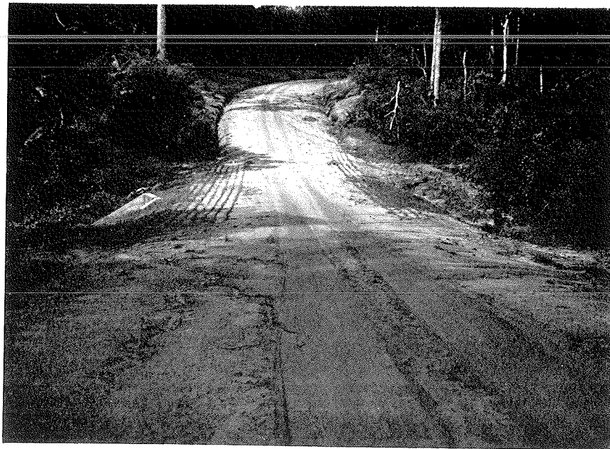
(A) Planting of grass to check erosion at a critical point—a shallow embankment on the road from Mamfe to Ikom, in the Southern Cameroons
