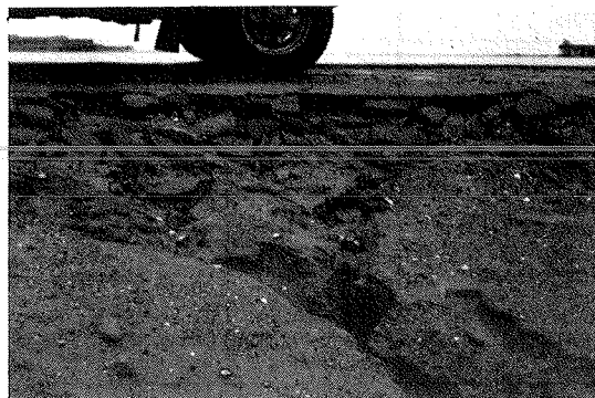
Breakup of bitumen stabilised road verge by traffic and rainwater erosion. Sand fill embankment. Zone IV. Trucial Coast
