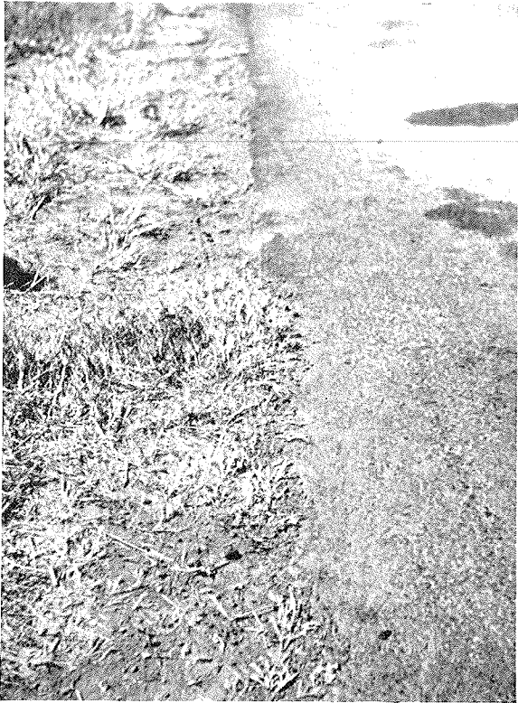
(B) Couch grass ( Cynodon dactylon ) encroaching on bituminous surfacing, on the Essexvale to Bulawayo road, Southern Rhodesia
