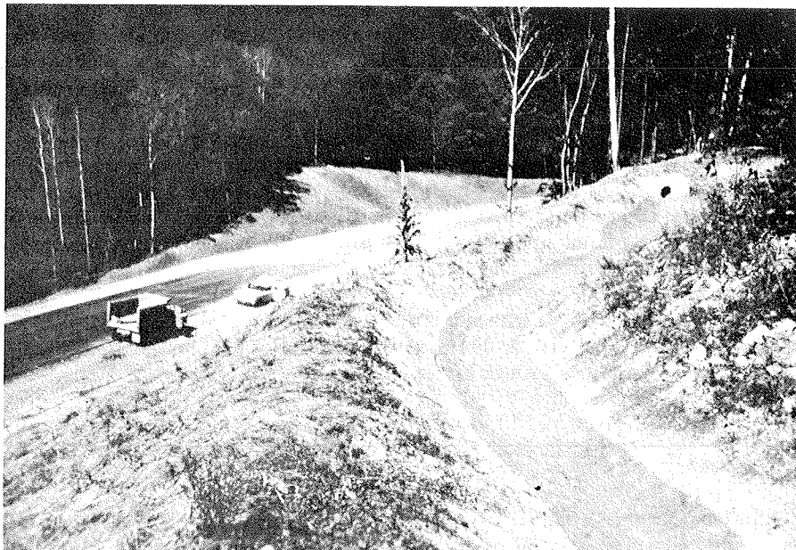
Interception at top of cut slope carries water to down drain and reduces slope erosion.
