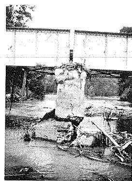
Figure 24. Front view of cracked pier shaft and broken pier footing.
