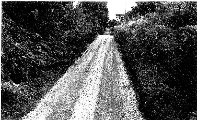
Fig. 26. Two extremes—above, a well constructed and maintained ditch; below, a ditch completely overgrown with weeds and brush.
