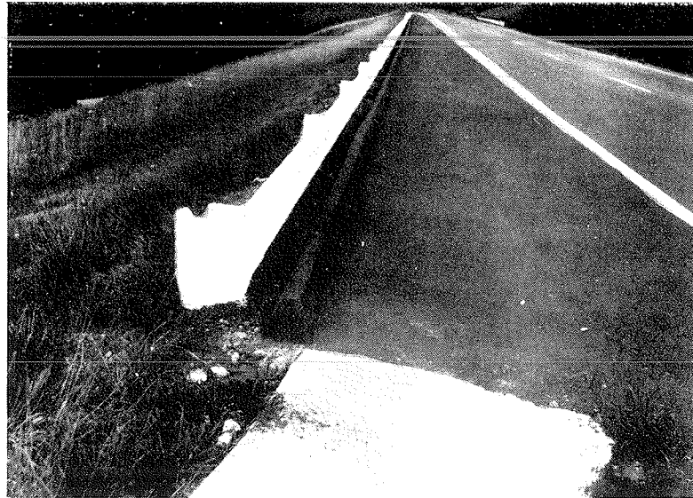
Fig. 10. This curb contains water from the long grade, so it will not destroy the side slope. Outlets both at the end of the curb and midway up the hill carry water safely to the foot of the slope.
