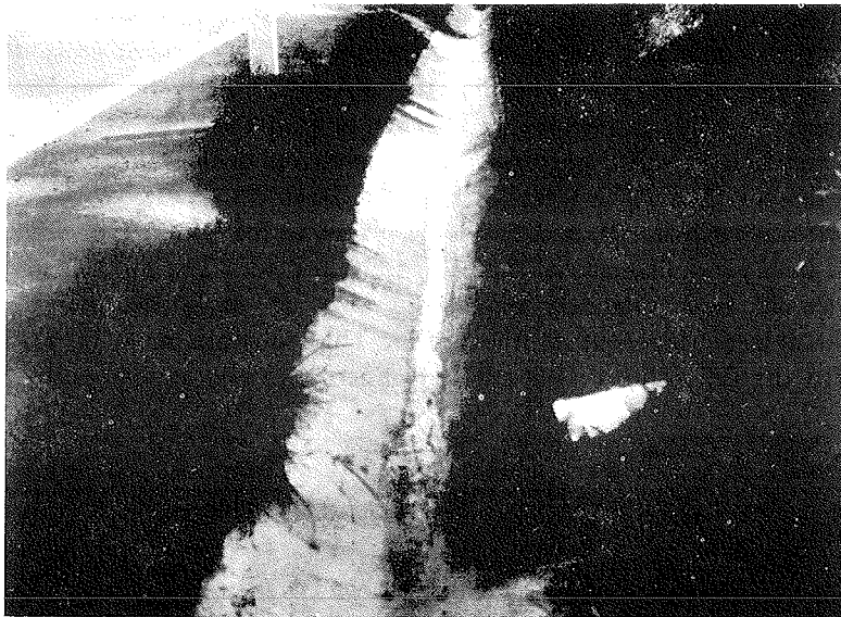
Fig. 12. Subdrains in the slope on the right keep the soil dry and stable. Notice the water in the ditch from the subdrains even during dry weather.
