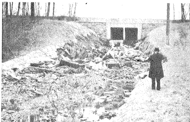
Same channel as above photo showing failure one year after construction. Foundation was not stable, undermining riprap.
