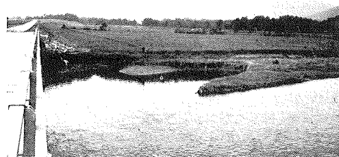
Figure 17. Enlarged scour hole upstream from Chemung River bridge in Waverly, N.Y.
