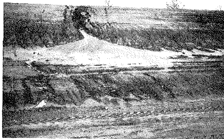
Care must be taken to control erosion and sediment during construction or large volumes of earth will be washed downstream.
