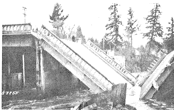
During unusual floods, channel banks erode and channel beds scour. Piling become exposed and some piers fail because of scour and inadequate foundations.
