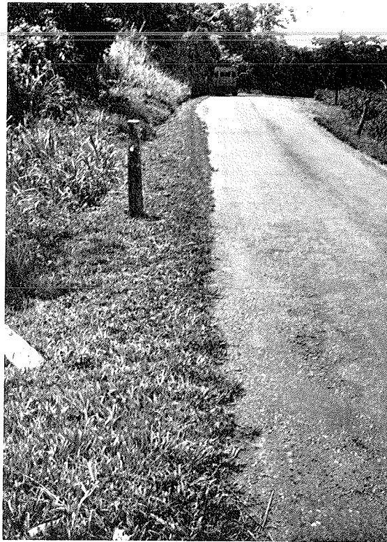
(A) A length of road in Western Nigeria, where the edge of the bituminous surfacing is protected by grass
