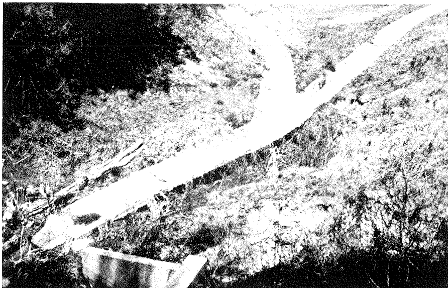
Rigid channels are vulnerable to undermining from splash and overflow, particularly on curves and channel confluences.
