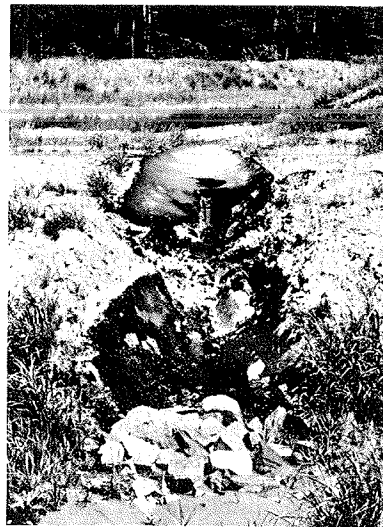
Figure 4. Asphalt lining of steep ditch along I-91 failed during first season.
