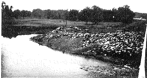
Figure 16. Remnants of earthfill spur dike near Chemung River bridge near Lowman, N.Y.
