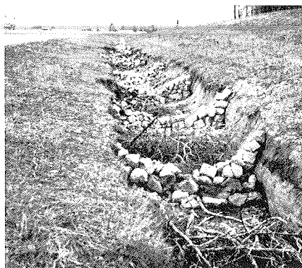
An eroded gutter is a costly maintenance problem and a safety hazard.
