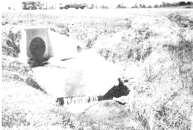
Scour at a culvert outlet can cause both culvert and embankment failure. Head-cutting from downstream can cause a similar failure.
