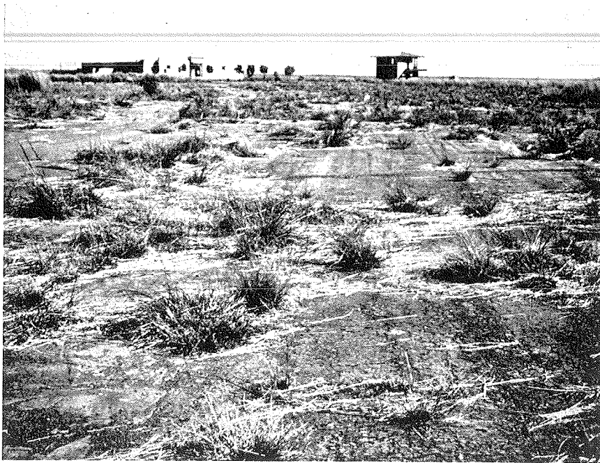
(A) Grass growing through an old, unmaintained, soil-cement pavement at Norton Airfield, Southern Rhodesia
