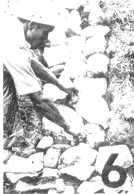
Figure 52. Riprap Down Channel (Indonesia).
