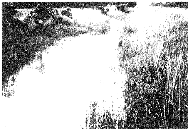
Figure 36. Standing Water in Roadside Ditch (Honduras).
