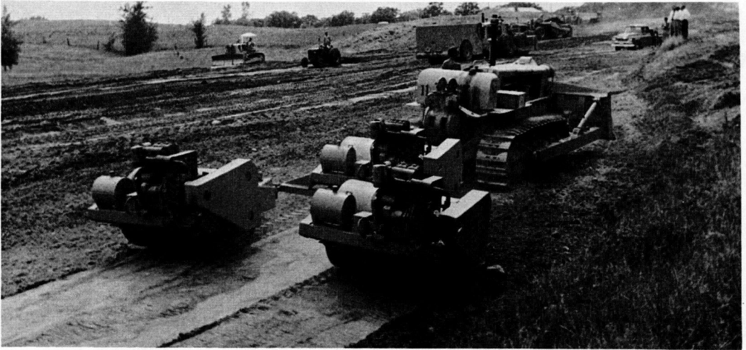
Figure 124. More than one type compactor are often employed on a project. Here a combination of three single-unit towed-type vibratory rollers and a heavy-duty pneumatic-tire roller are seen on the same project.
