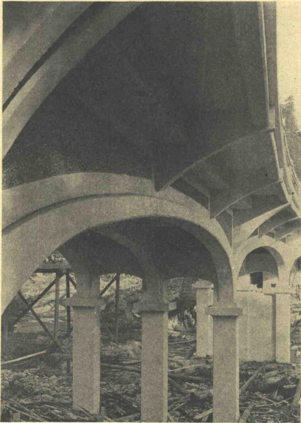
Figure 22. A Close Up of the Underside of the Structure Shown in Figures 20 and 21
