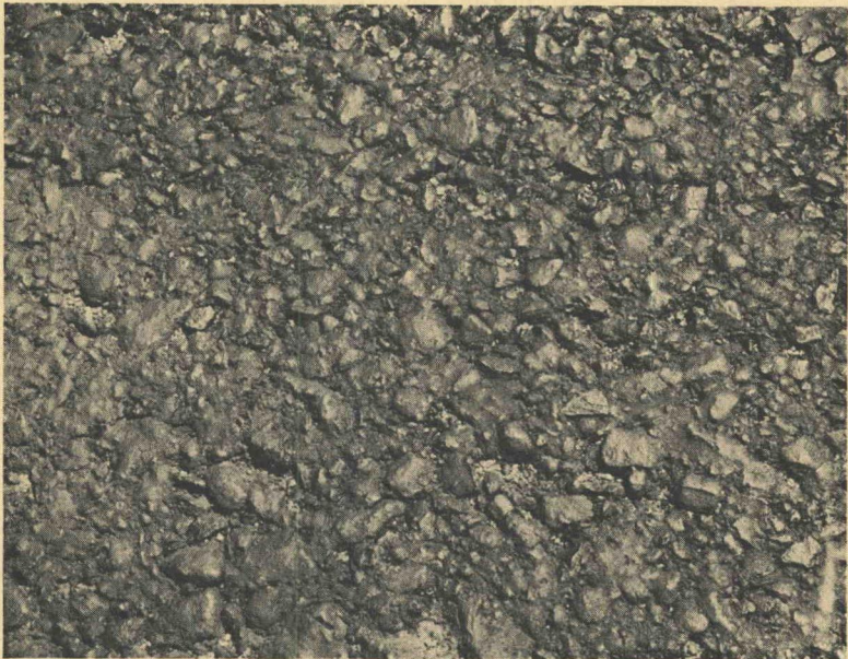
Figure 5. Close-Up of Pavement Surface Shown in Figure 4
