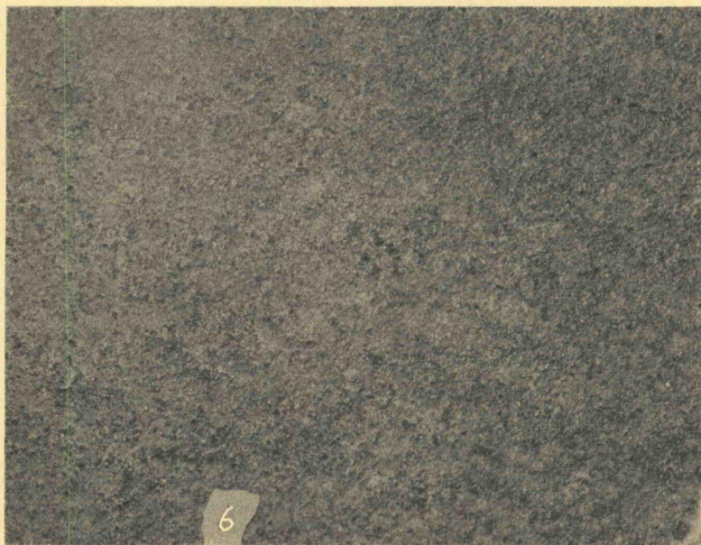
Figure 7. Close-Up of Pavement Surface Shown in Figure 6
