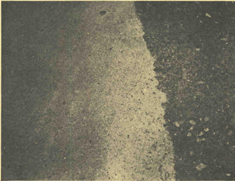
Figure 15. Close-up of edge of above patch (Fig. 14) where it is zero inch thick. No scaling after seven years of "Main Street" traffic.
