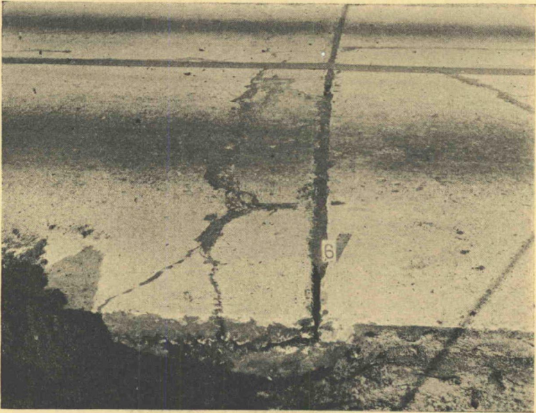
Figure 10. Three-and-one-half-inch resurface on four-inch base with widening section eight inches deep. Joint space not cut through to old base. Resulting underspall faulted joint and caused joint breakage under loads.
