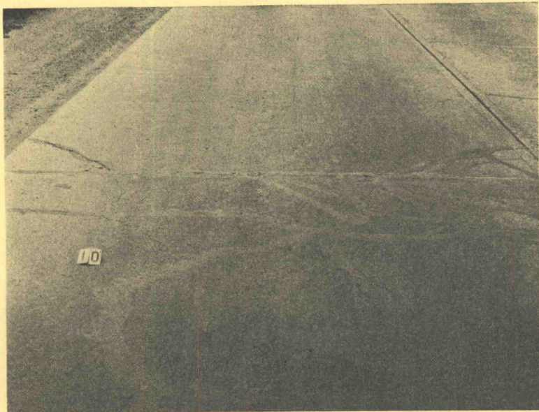
Figure 12. Breakage at an expansion joint which had faulted one-inch
