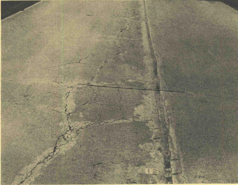
Figure 8. Five-inch resurfacing increasing to seven inches over edge of old base. Center joint having no mechanical bond nor tie bars. Mesh in outer 4 feet of old slab only. Longitudinal cracking 2 to 3 feet from center joint because of lack of bond across joint. Badly broken base.
