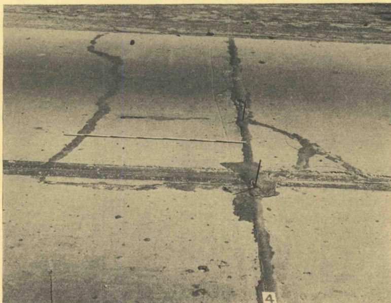
Figure 11. Longitudinal crack (marked by pencil) over a dowel not placed parallel to surface of slab. Corner crack also starts over dowel. Joint itself is properly placed. Old base not broken.
