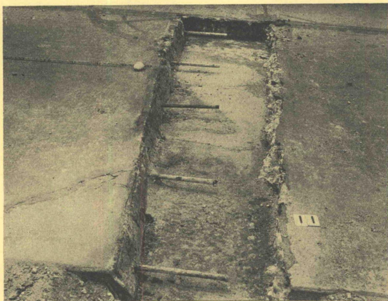
Figure 13. Above joint (Fig. 12) with broken concrete removed. Note sloping face, which caused the faulting. In this case, as in others noted, dowels did not prevent faulting.
