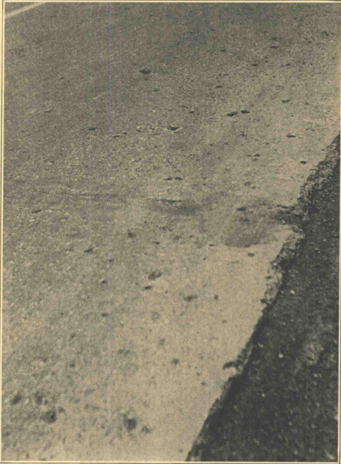
Figure 3. Pits in Concrete Pavement Due to the Presence of Soft Stone in the Coarse Aggregate
