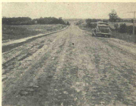
Figure 26. General view of surface on 8 per cent soil-cement machine mix base. Raveling occurred after priming but the prime coat kept it from becoming excessive. Several weeks later the left half was primed with TC-2 and the right half with MC-1. Missouri photo.
