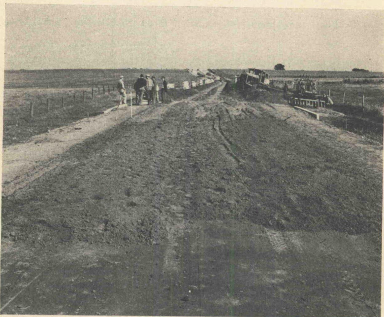
Figure 23. A typical turn-around, the mixed material windrowed on either side of the next increment, and the cement ready to be placed. Illinois photo.
