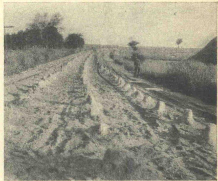
Figure 3. Cement sacks were placed at a specified rate and emptied prior to spreading with a motor grader. Missouri photo.
