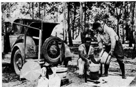
Figure 6. Sampling of Soil from the Roadway for a Relative Compaction Test. Left to right are Orchard post hole auger, sample, scale and rubber bag. The volume occupied by the sample is being measured by the water displacement method. A thin rubber bag (Figure 7) is first placed in the test hole to prevent the water from soaking into the adjacent soil.
