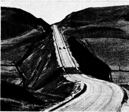
Figure 15. A 900,000 cu. yd. embankment, 80 ft. High, Constructed in 1933 and 1934 on the American Canyon Project in California. No appreciable settlement to date (November, 1938).
