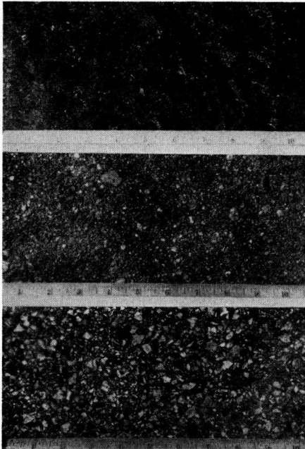
Figure 3. Close-Up Photographs of Bituminous Surfaces in Kansas. (Upper) Glazed Sandy Bituminous on Kansas Route 96, (Center) Sandy Bituminous on U.S. 77, and (Lower) Chat Rock Chip Bituminous on Kansas Route 99.
