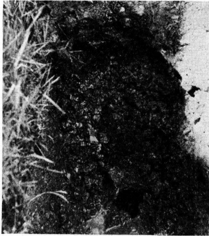
Figure 8. Two-inch crushed stone backfill entirely clogged with soil at pipe level and nearly so above pipe.
