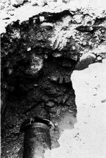
Figure 10. Backfill of broken field stone choked with soil.
