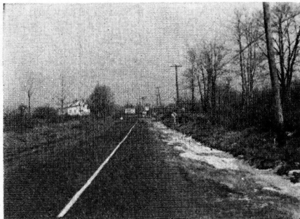
Figure 3. Seepage out of Gentle Hillside. Note the reference stakes for proposed underdrain.
