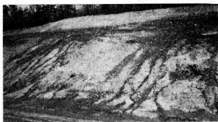
Figure 6. Seepage Line at contact between pervious sandy till and impervious clayey till. Irregular seepage line at irregular pervious lenses. Two subsurface drains now collect 5 g.p.m. each.
