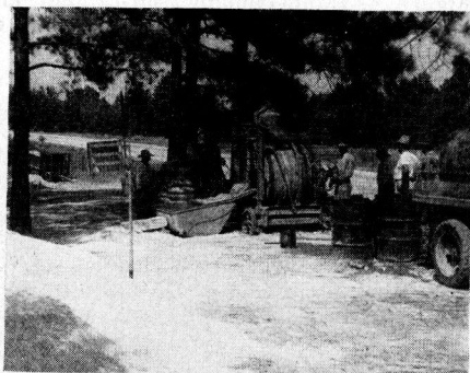
Figure 3. Mixing soil and cement. Soil stockpile in left foreground is disintegrated sandstone.
