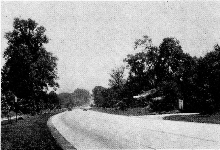
Figure 7. A strip of plant mixed bituminous pavement with coarse aggregate serves as a transition between the turf shoulder and the concrete. Motorists are warned that they are leaving the pavement by the sound of tires on this "black top." Note clean edge of healthy turf and lack of the rut commonly found along traffic lanes less than 11 ft wide.
