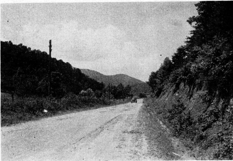
Figure 3. A Federal-Aid Highway Constructed about 1924. Note lack of shoulder pitch and clogged drainage ditch resulting in saturated subgrade under both pavement and shoulder. Shoulders partly weed covered, soft and unsafe in spring when frost is leaving ground.
