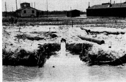
Figure 8. Pipe Discharging Water into Sump for Ponded Area Test.
