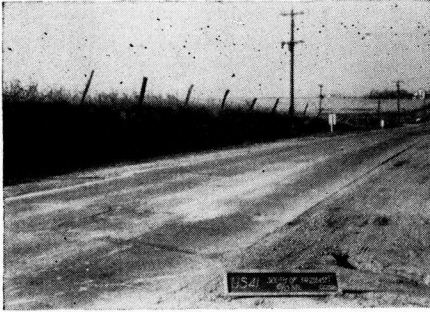
Figure 8. Ground View of Maintenance Patching and Pumping Slabs in Cut Section Shown in Figure 7
