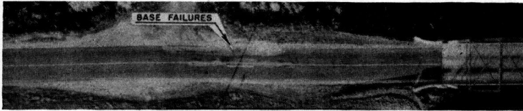
Figure 4. Base Failures on Rock Asphalt Pavement
