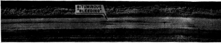
Figure 3. Fat Spots Caused by Bleeding of Bituminous Surface Treatment
