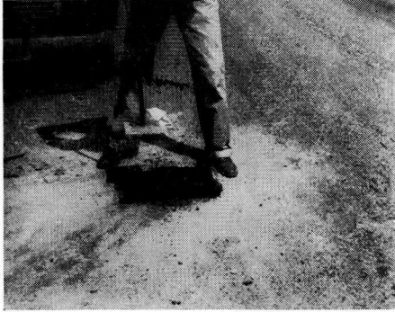
Figure 8. Patching the Opening. This was carefully done to prevent infiltration of moisture. The top 4-in. of the patch consisted of cold-patch material.
