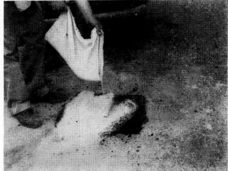
Figure 10. Sand Spread Over Fresh Patch to Blot Any Excess of Bituminous Material
