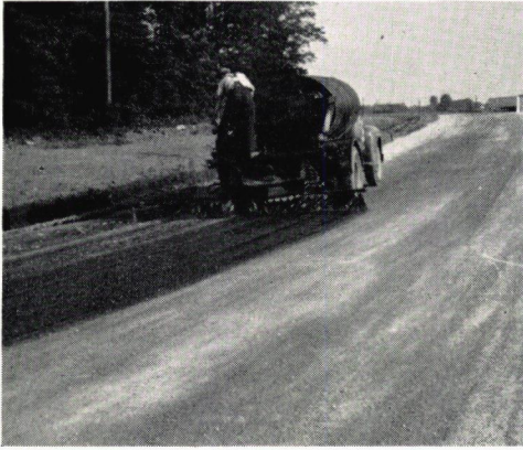
Figure 11. Appearance of the finished dense-graded base at the time priming for the bituminous pavement was started.
