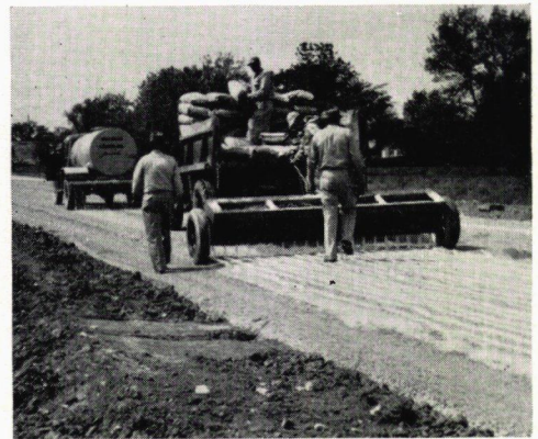
Figure 7. Water was applied to thoroughly wet the stone prior to application of calcium chloride. This was done to assure an adequate moisture content and prevent segregation as well as facilitate manipulation during the mixing process that followed.
