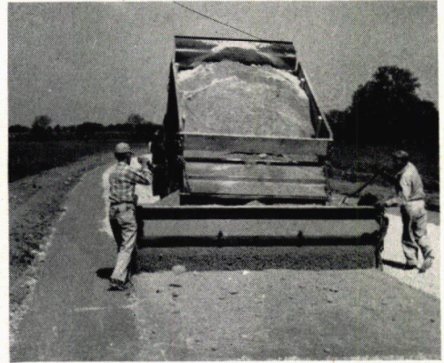
Figure 6. Placing finer aggregate for the dense-graded course over the crusher run material shown in Figure 5. Because of the insufficient quantity of material finer than the No. 200 mesh in the first stone placed, it was necessary to add fines which are normally sold for agricultural lime from this quarry. This fine fraction represented 25 percent of the total aggregate.
