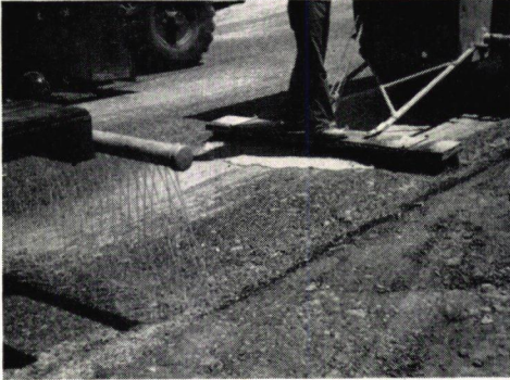
Figure 4. Watering, brooming, and rolling on the waterbound construction. Note slurry in front of the broom.
