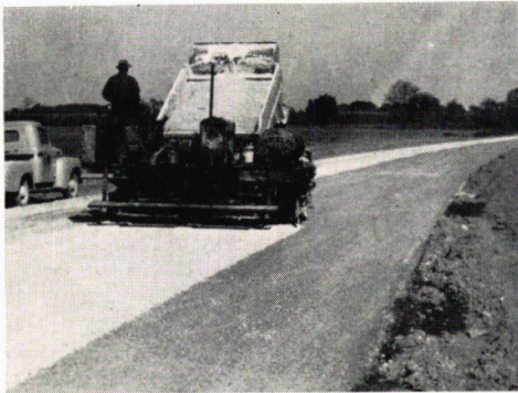
Figure 5. Spreading the coarser of two aggregates used for the dense-graded base course construction. This stone was crusher run through a 1-in. screen with approximately 3 percent passing the No. 200 screen.
