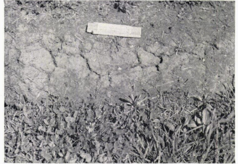
Figure 3. Map cracking in soil.
