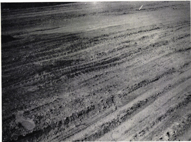
Figure 2. Soil which by old rating system would not require treatment. Nonplastic; minus No. 200, 35 percent; total volume change, 16 percent; maximum density, 79 lb. per cu. ft.
