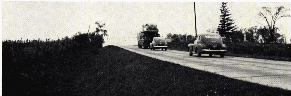
Figure 1. Short sight distance, narrow width and appearance of the pavement before resurfacing.
