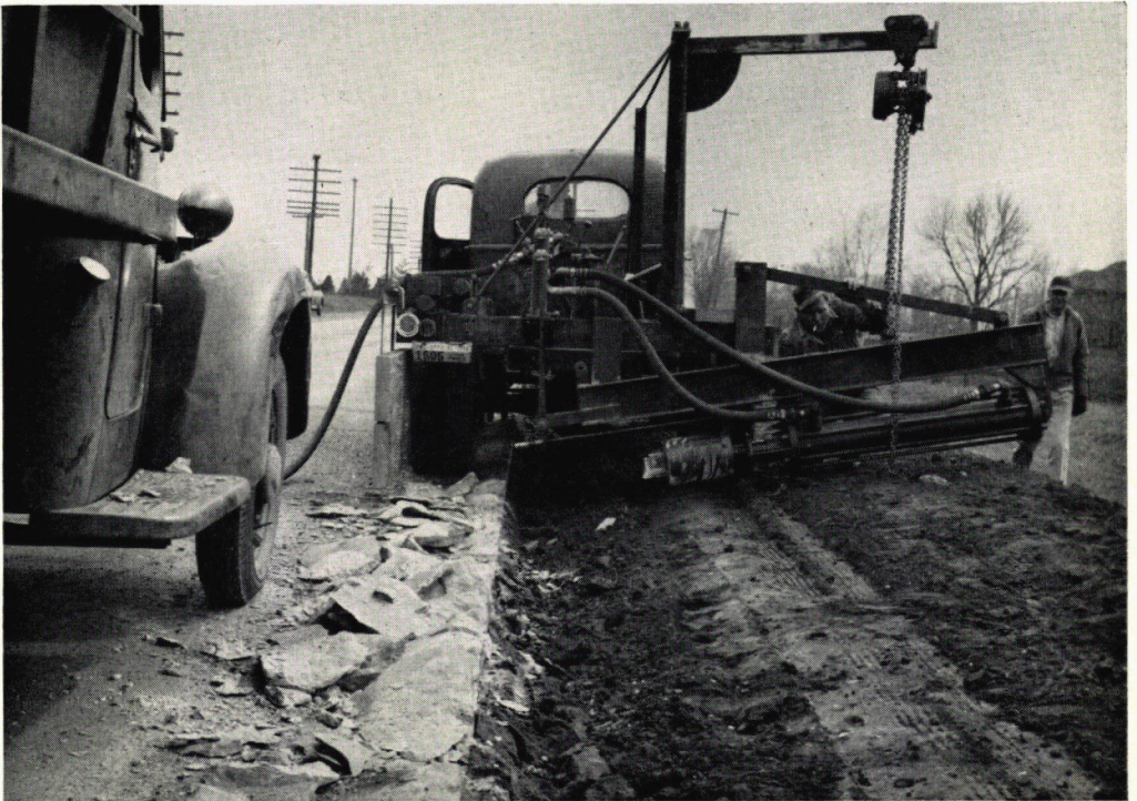
Figure 4. Machine developed by C. L. Gleason, construction engineer, Iowa State Highway Commission, to remove all integral curb before resurfacing.
