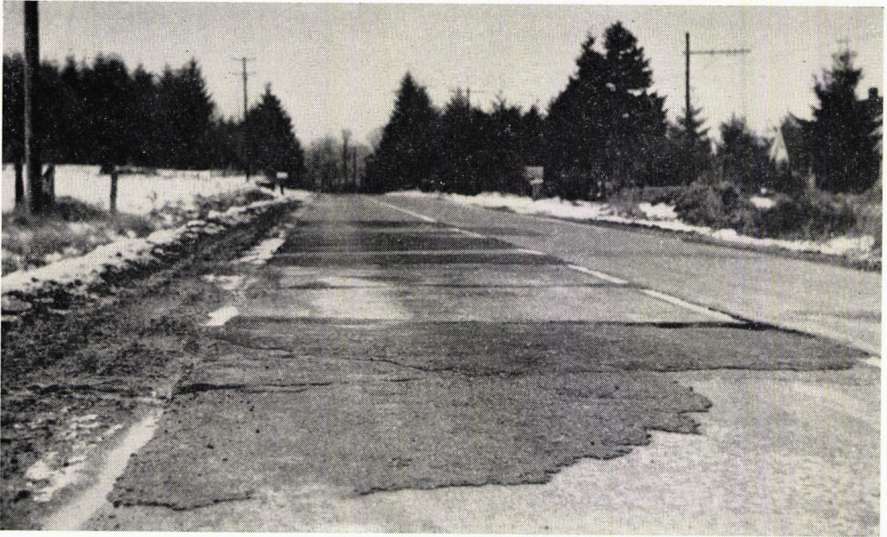
Figure 7. Condition of pavement before start of work.
