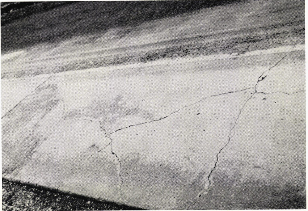
Figure 9. Section of pavement broken by compactor.
