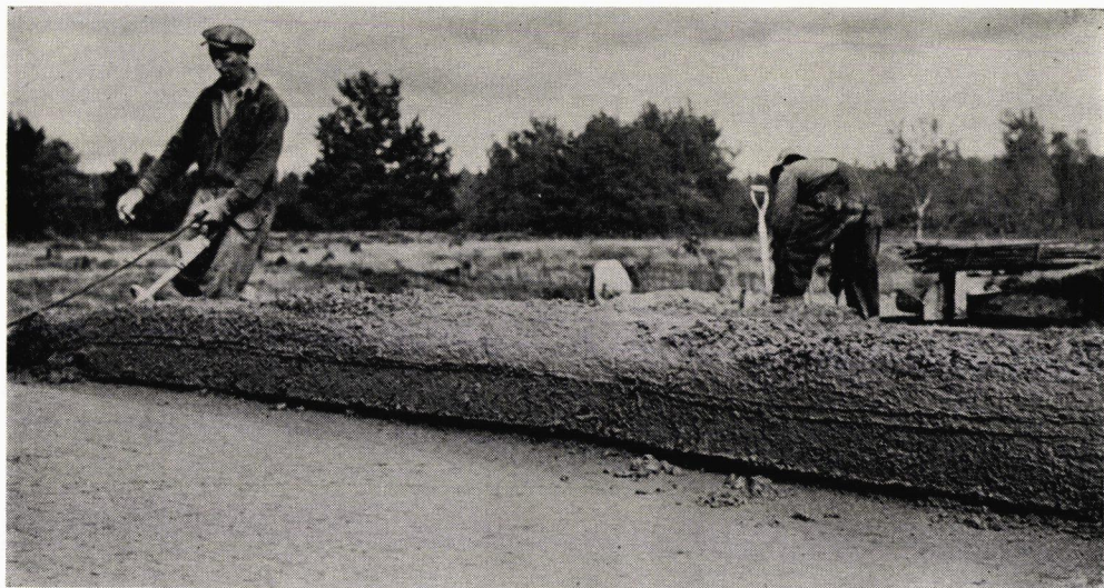
Figure 22. Typical appearance of concrete containing added fines.
