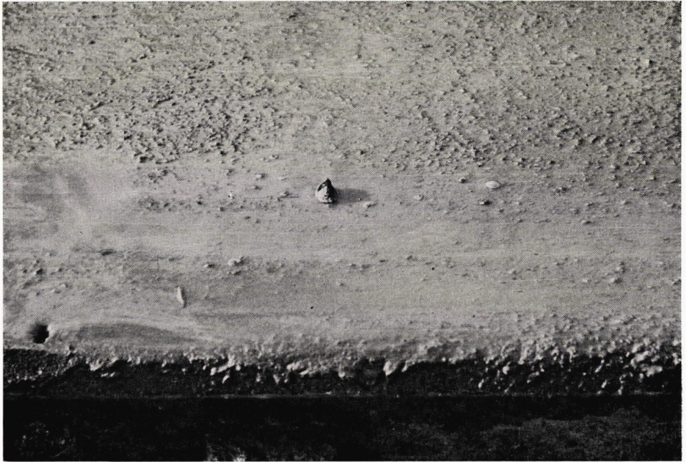
Figure 24. Bleeding of concrete containing limestone fine and coarse aggregates.
