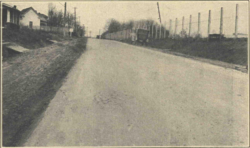
Figure 3—Wet Cut with Pavement Failures
