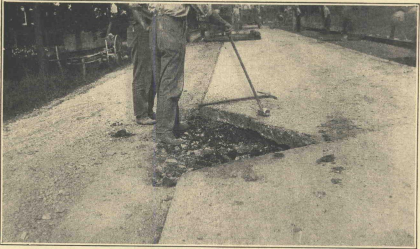
Figure 31—Maintenance on Road No. 108-DeKalb, Sycamore, Ill. Preparation for replacing corner failure with concrete
