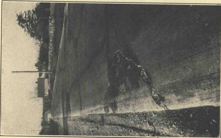
Figure 13—Corner breaks, Road No. 21, Town of Norton, Mass.
