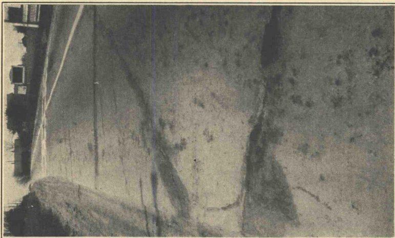
Figure 9—Raveling of crack 6-8-6 section, Road No. 193, Pennsylvania
