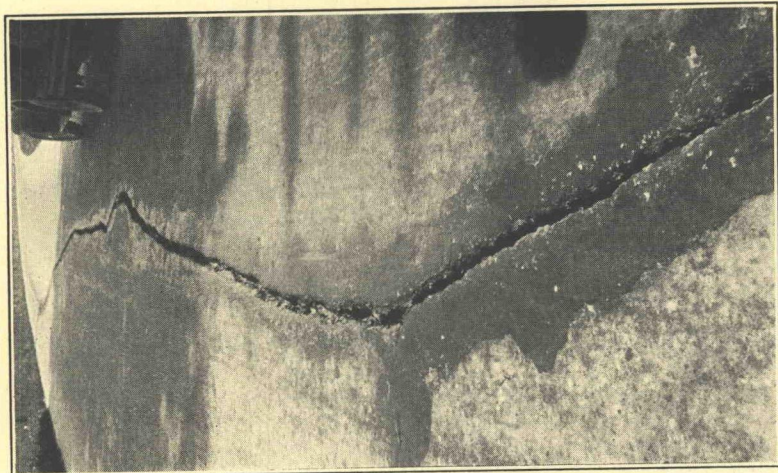
Figure 12—Separation of slabs 7 inch section, St. Clair Co., Michigan
