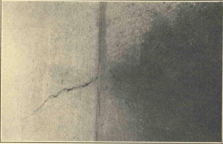
Figure 55—Meeting of closed crack in reinforced slab with open crack in plain slab, Milwaukee Co., Wis.
