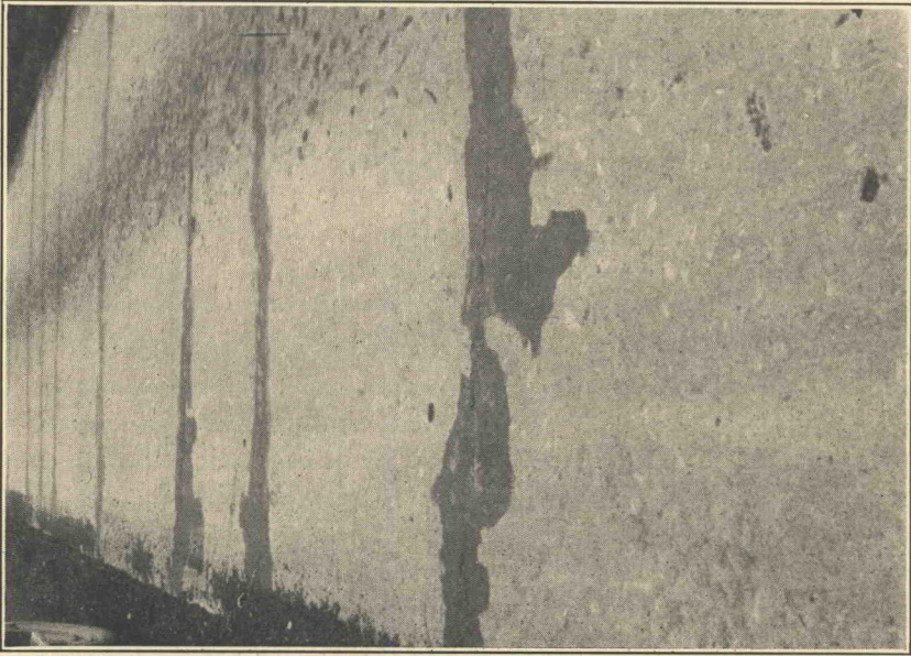
Figure 22—Excessive transverse cracking in narrow slab laid on peat bog subgrade. (Celeryville Road No. 88, Ohio.)
