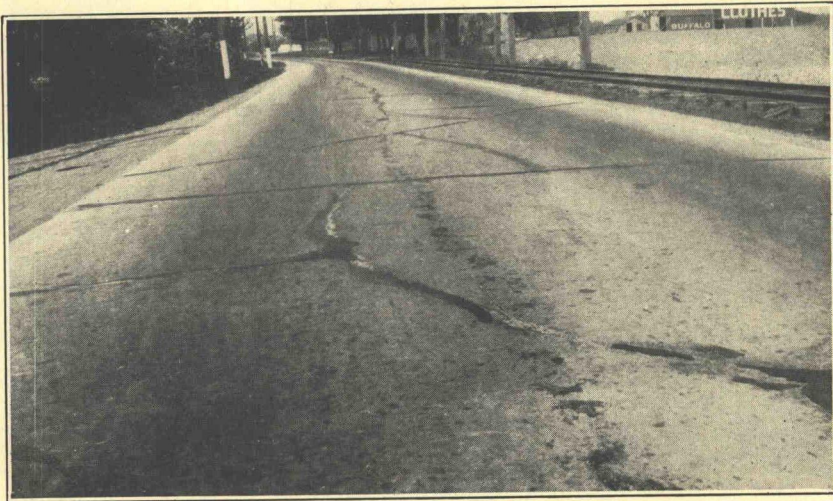
Figure 6—Cracking in Road No. 193, Pennsylvania
