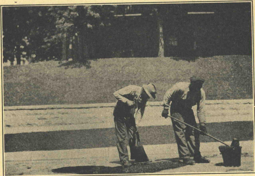
Figure 67. Light Patching Is Done with Thin Layers of Bitumen and Aggregates Applied Separately
