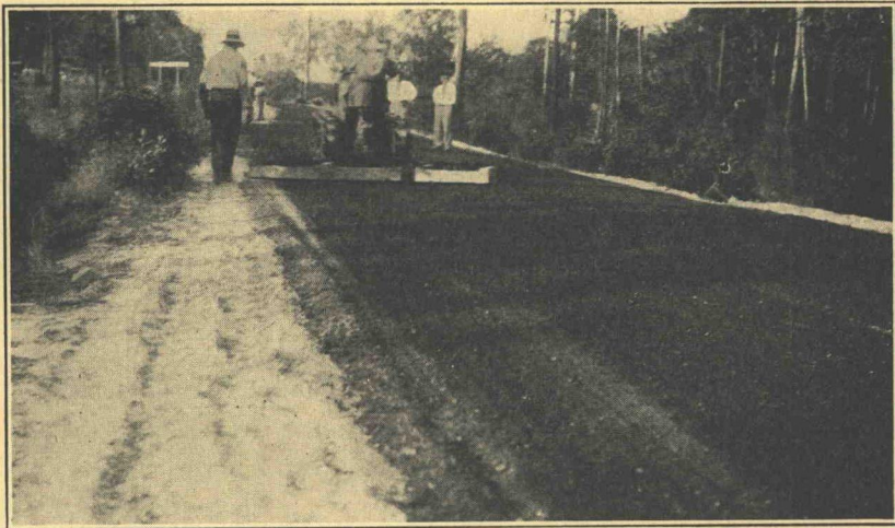
Figure 72. Mixed-in-Place Bituminous Surface, Fine Aggregate Type. Final Dragging of the Mixture Before Compaction with a Power Roller. North Carolina
